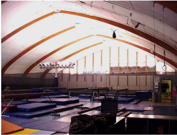
Existing 146 - 1000 watt Metal Halide fixtures. Replaced with 76 - 1000 watt BEST Lights MH-ISP Twice the light levels with 1/2 the fixtures.
