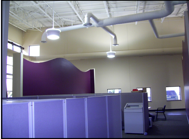
Office: 6,300 sq. ft. 27' high / 10 -750 Watt Pulse Start MH-XL-DIG (62% indirect 38% direct) 1.2 Watts per sq. ft. general lighting 35 FC
