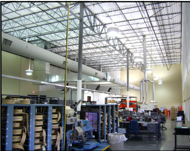
Inspection: 5,800 sq. ft. 27' high / 15-750 Watt Pulse Start MH-XL-DIG (62% indirect 38% direct) 1.98 Watts per sq. ft. 90 FC
