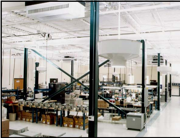
Accumentrics Inc. 20,000 sq. ft. with 20' ceiling; 400Watt MH-DIC ; 60 FC
